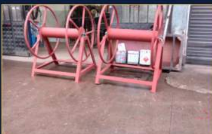
Fire hose reel assembly
