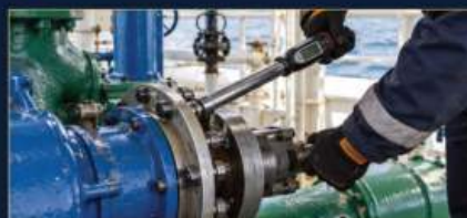
Pump service onboard
